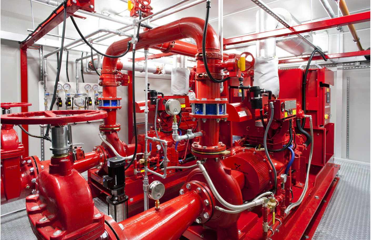
Fig 1 - An example of the interior of a typical packaged pump house
